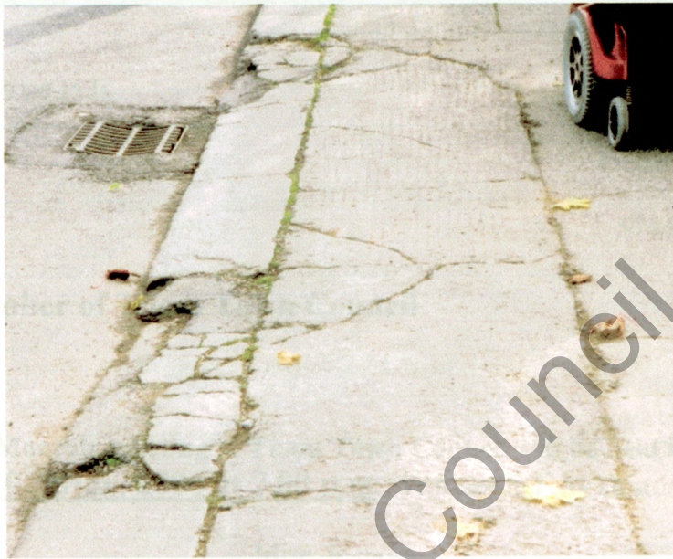
No way to get on pavement at crossroads
