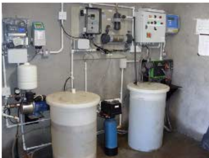
Photograph 3-3: Sodium Hypochlorite Disinfection System.
