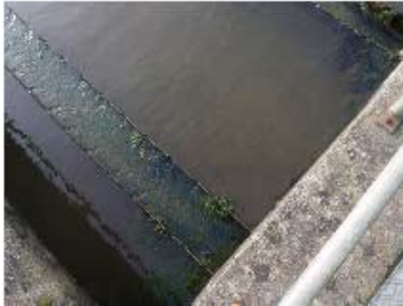
Photograph 3-4: A poorly operated clarifier (note the excessive algal growth and overflow of water into the clarification channel).
