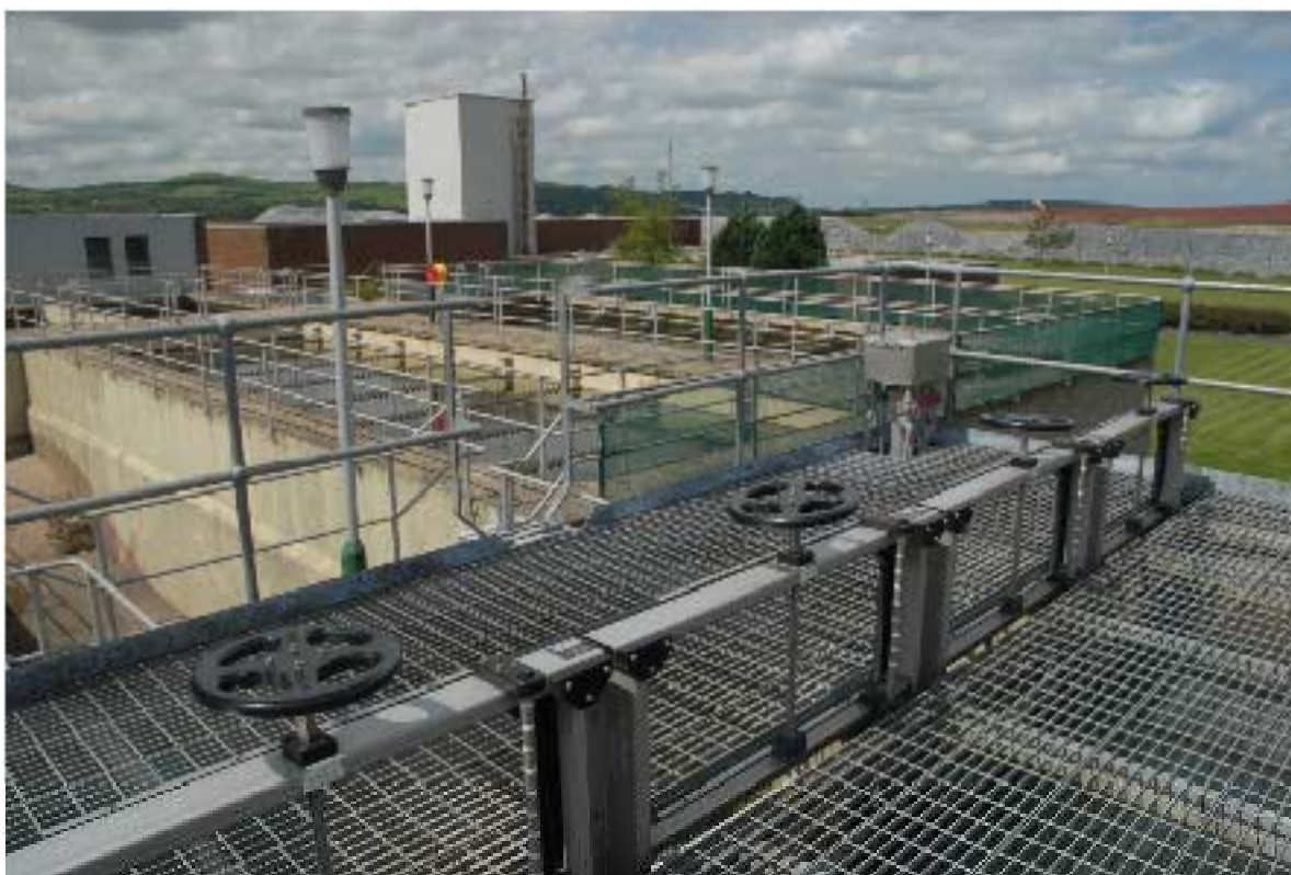
Photograph 2-1: Foynes (Shannon Estuary) Water Treatment Plant (Co. Limerick)
